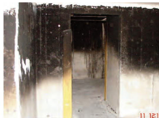
Figure C-7: Interior View of Burn Prop
